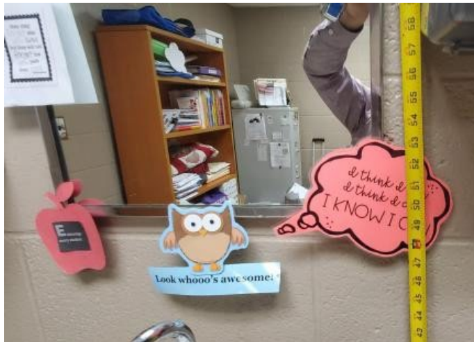
As Built: The mirror is mounted too high.
